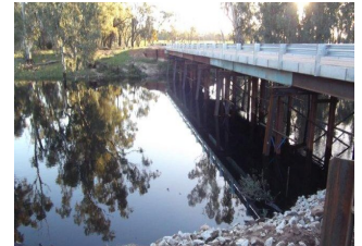
Photo of new bridge over the "Thule Creek" taken 17th March 2012. Unfortunately black water is currently coming out of the Koondrook Perricoota Forest with critically low dissolved oxygen levels (1.68 mg/L)
