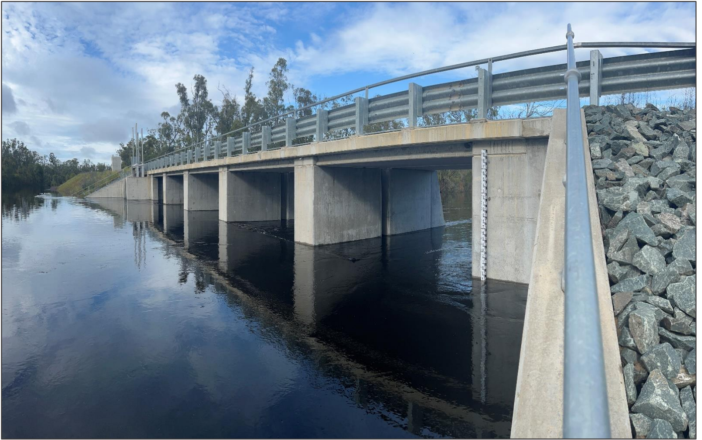
Figure 4: Barbers Ck regulator showing the water level (5.816m) above to 2016 water stain mark
