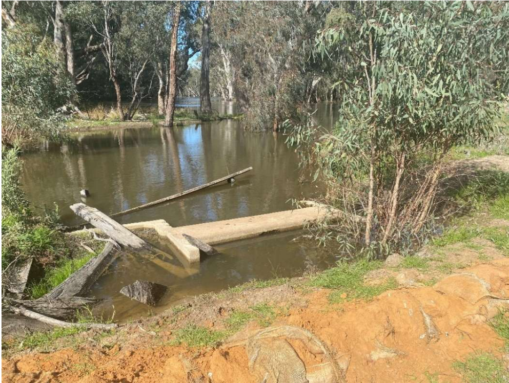
Figure 13. Current inactive regulator offtake from the Little Murray River on Gonn Station.
